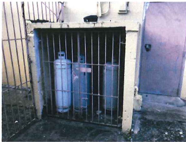
Figure 1 – Gas tanks are loose
