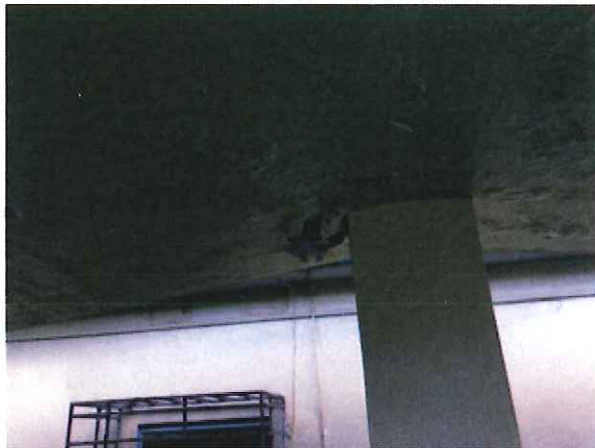
Figure 2 – Exposed rebar at gazebo
