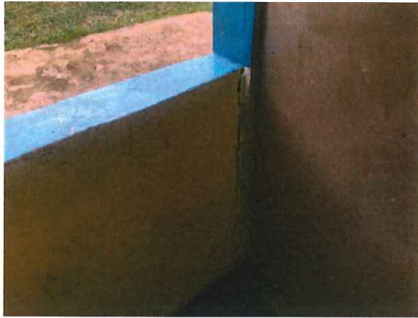
Figure 10 – Low wall crack
