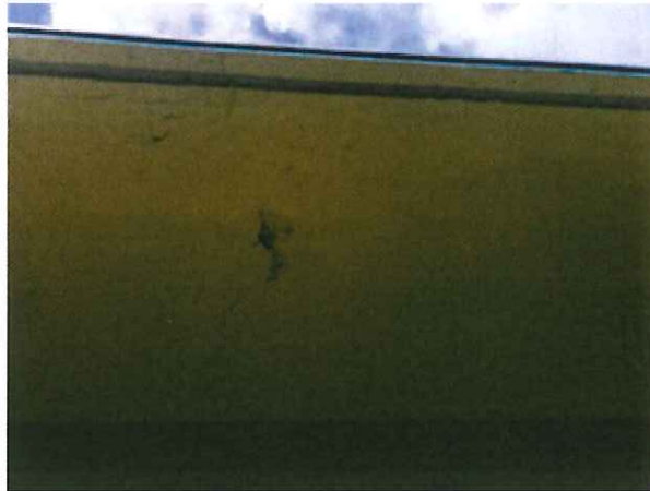
Figure 6 – cracks at ceiling
