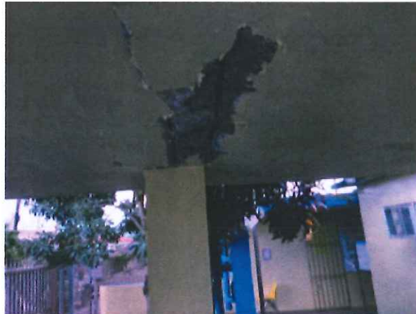
Figure 4 – Exposed rebar and spalling of concrete ceiling at gazebo
