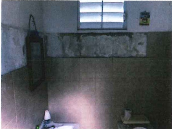
Figure 11 – Wall tile fall after seismic event
