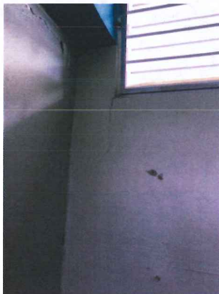
Figure 5 – Cracks at wall
