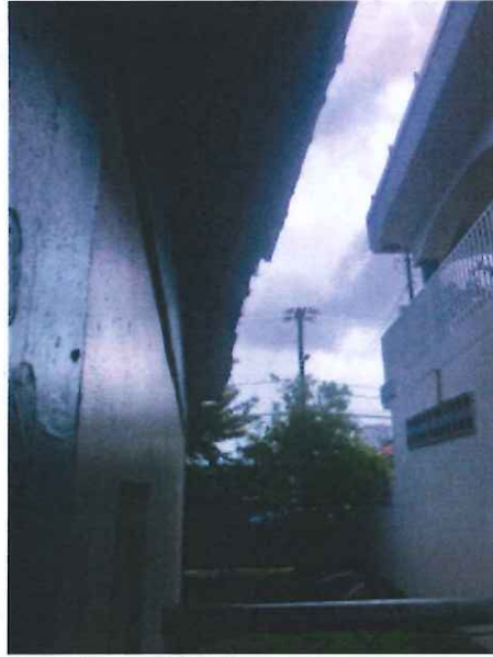
Figure 12 – Spalling of concrete ceiling overhang
