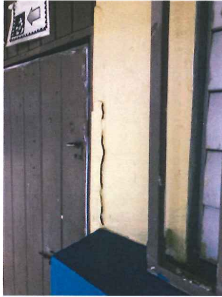
Figure 8 – Cracks at wall door
